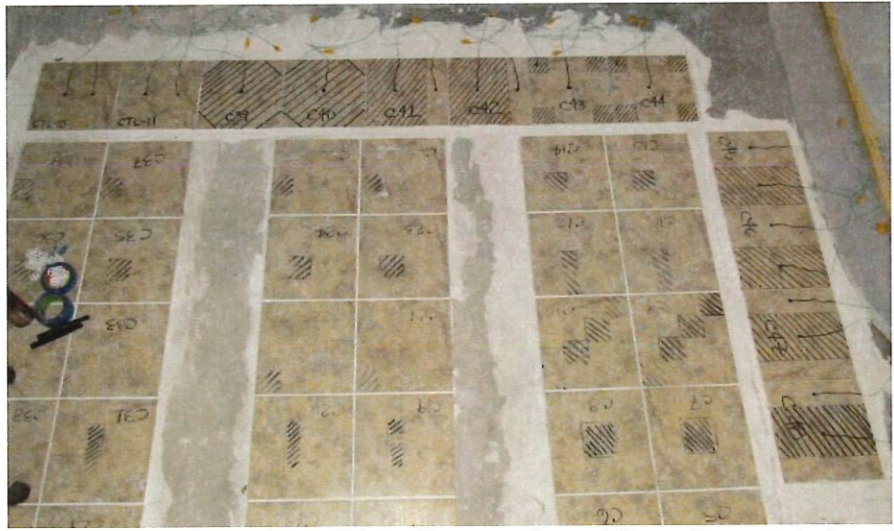
Photo 2: Tile tap test of floor tiles with hollow portions either above or below the thinset. Tiles on the left have nonbonding below the thinset while tiles on the right have nonbonding above the thinset
